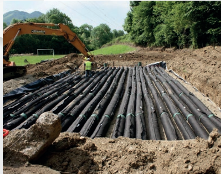
The rows of Advanced Enviro)Septic pipes
